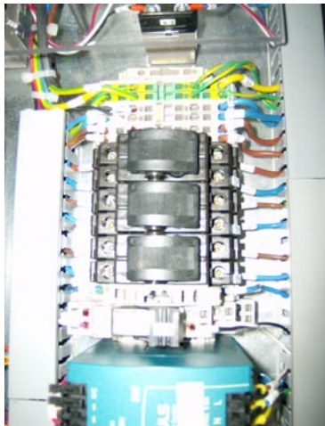
Figure A2: Circuit Breakers (In Control Enclosure)
